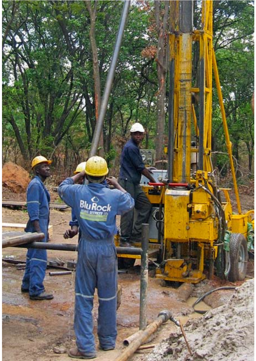
Exploration drilling with a CS1000 core drill rig at Muliashi, Luanshya Mines.
